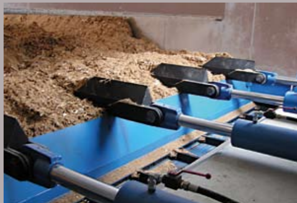
Typical biomass walking floor
