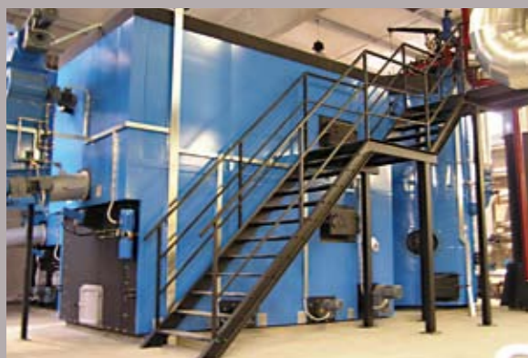
2MWth Biomass boiler
